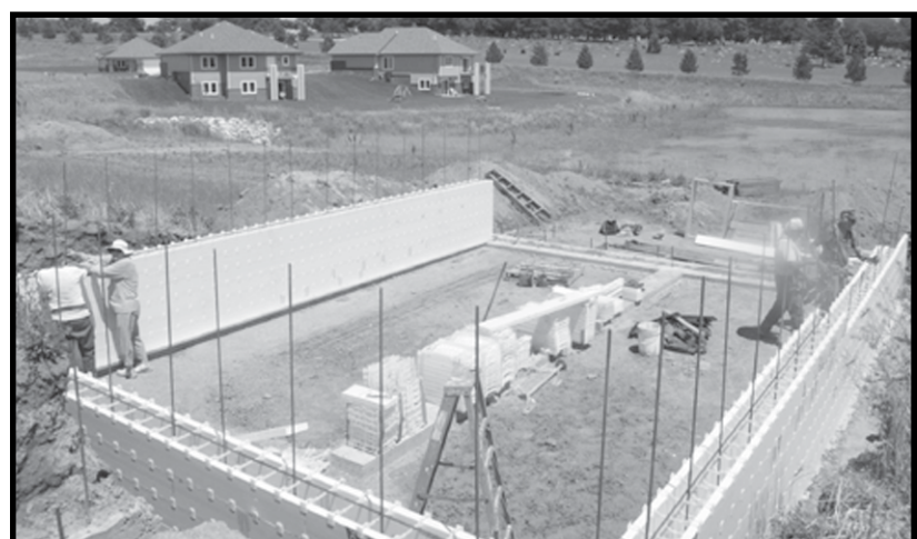
Volunteers assisting with the current Habitat for Humanity home had ideal weather conditions last week as they installed the lite form walls for the house.
